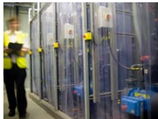
OSEC disinfection dosing pumps at Hampton Loade Water Treatment Works
