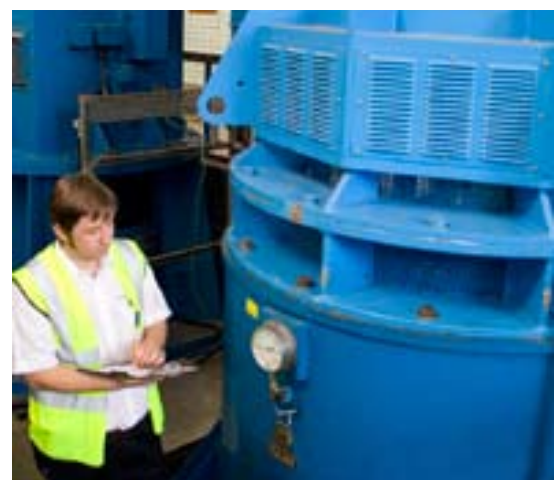
High lift pumps at Hampton Loade Water Treatment Works, refurbished with high efficiency motors but retaining the existing pump
