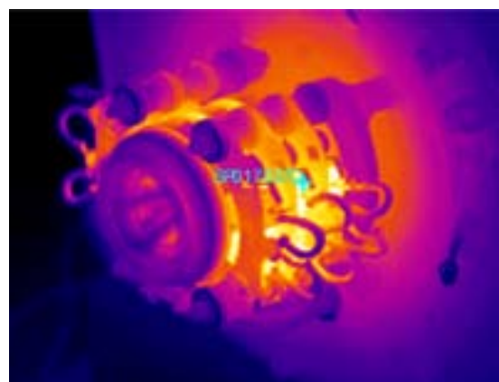
Thermography process - technology used to detect excessive heat, indicating potential failure of asset
