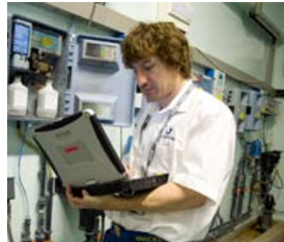
Water quality instruments at Hampton Loade Water Treatment Works
