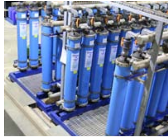
Complex treatment process example, the membrane plant at Seedy Mill Water Treatment Works
