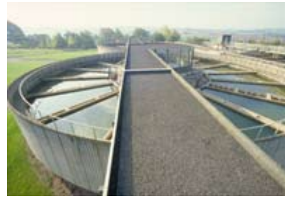
Clarification treatment process at Hampton Loade Water Treatment Works
