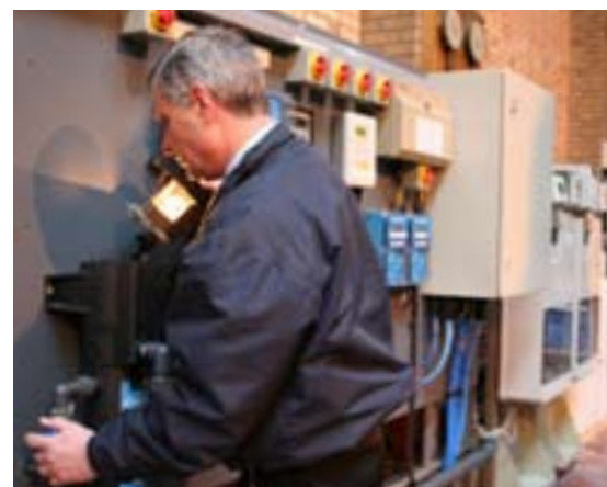
Water quality instruments at Seedy Mill Water Treatment Works
